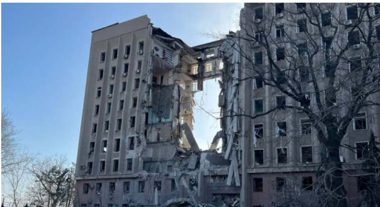
Results of the attack on the Mykolaiv Regional State Administration building.
